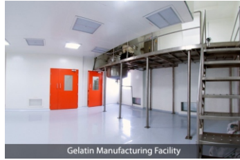
Gelatin Manufacturing Facility
